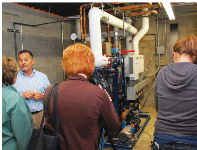
Mahomet IGA President Brooks Marsh shows reporters the store’s new geothermal unit at a media event held March 30, 2010.
